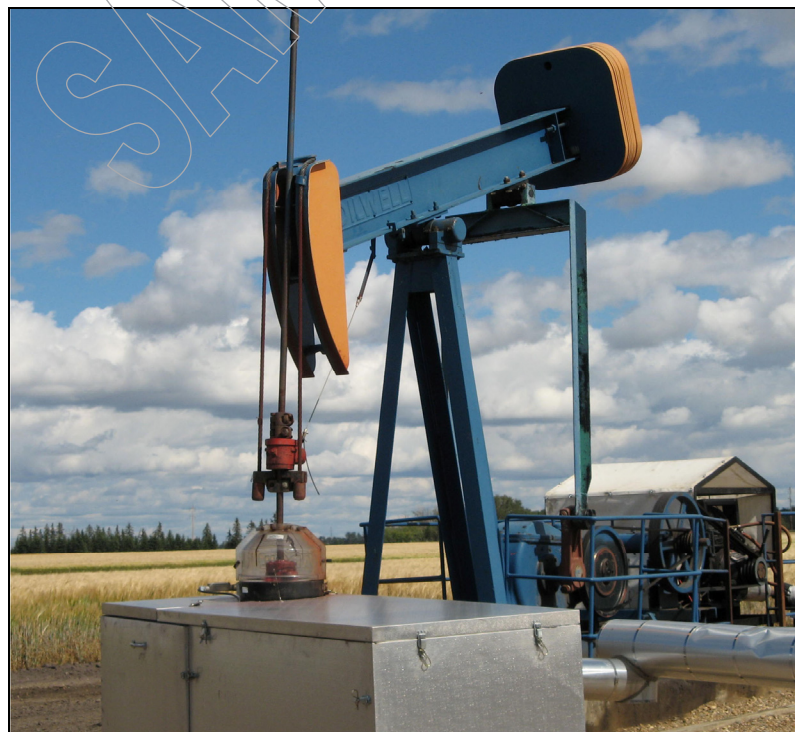
Figure 4 —Beam-Balanced Pumping Unit
